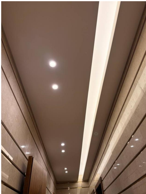
Figure 3 - Corridor Connecting Bedrooms Ceiling
