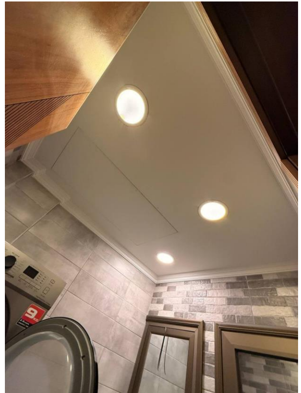
Figure 10 - Laundry Room Ceiling
