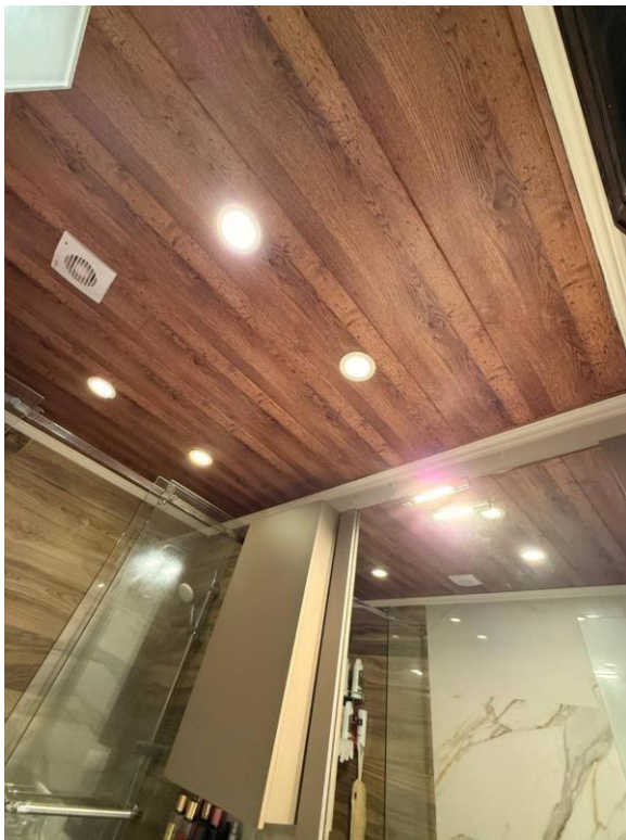
Figure 7 - Master Bedroom's Toilet Ceiling
