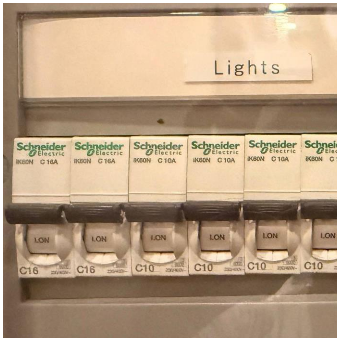
Figure 1 - Abed's Apartment Panelboard, Lights Section
