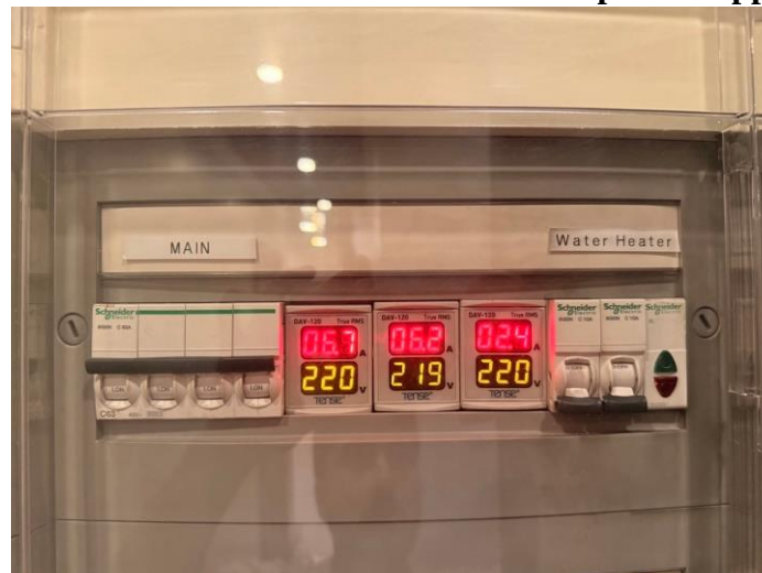
Home Distribution Panel-board - Three-phase Supply
