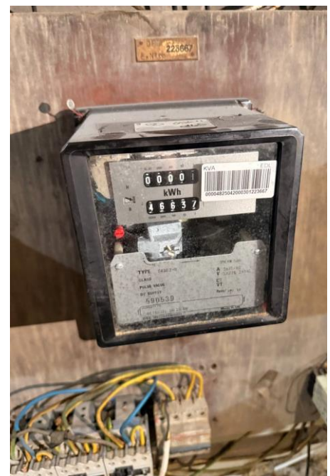
Figure 8 - Three-phase EDL meter serving Abdul Kader's apartment
