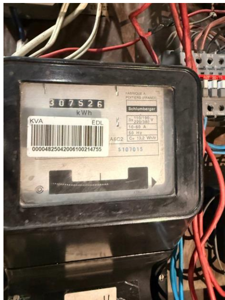
Figure 14 - EDL three-phase meter marked 220/380 V, 50 Hz
