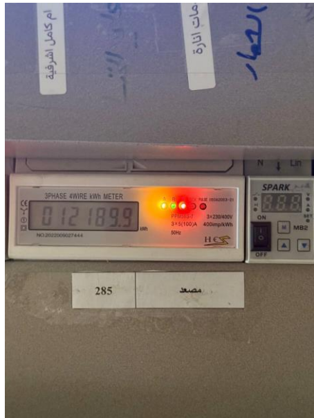
Figure 12 - Supplier Elevator meter: 3-phase, 4-wire, 3 x 230/400 V
