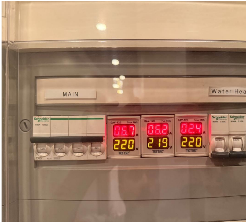
Figure 5 - Apartment Panel Board: Schneider four-pole C63; phase readings = 220/219/220 V (3-Phase)
