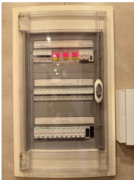
Figure 1 - Abdul Kader's Apartment Distribution Board
