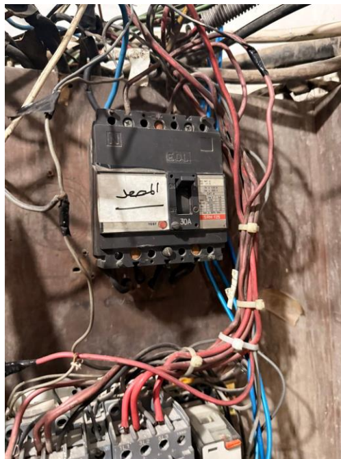
Figure 7 - Separate EDL elevator breaker, handle marked 30 A
