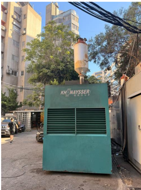
Figure 10 - Hashem Electric Distribution Generator Unit
